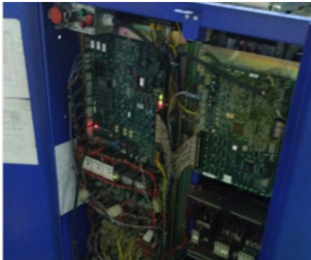
Electrical Adjustments & Maintenance of Non-SJEC brand
