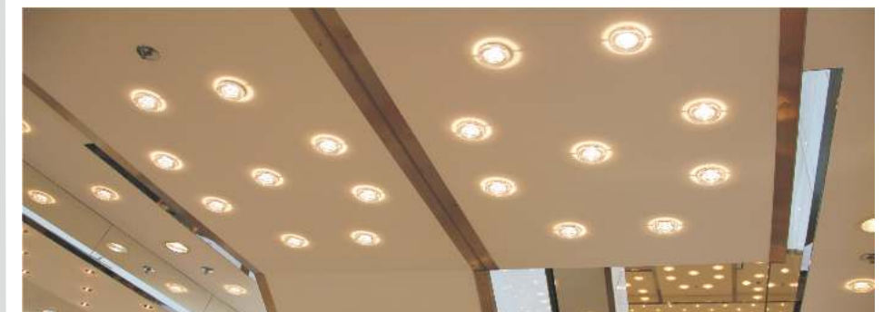
LED spot lighting
